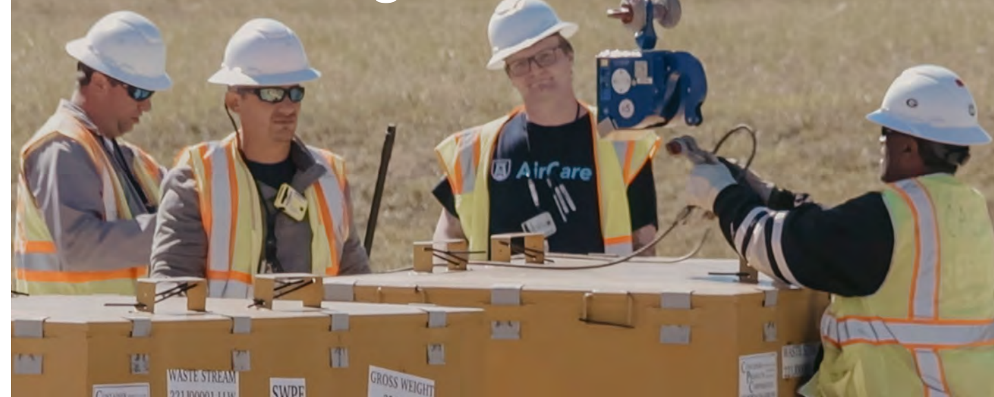
Alex Wilson, Ricardo Villalobos, Jonathan Alligood, and Calvin Sanders hook a low-level waste (LLW) box to the new remote release hook.
