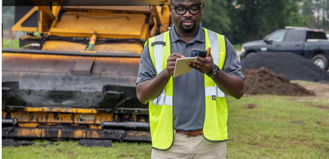
SRNS Senior Engineer Wisdom Hokey inspects the progress recently made during the paving of Road 4, one of the Site's most traveled roads.
