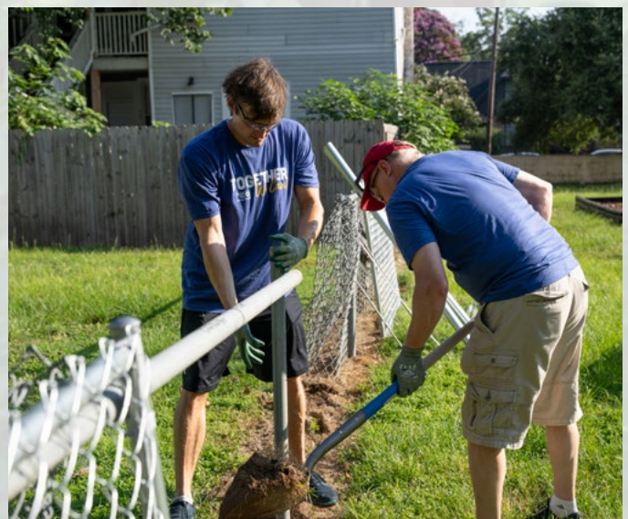
SRNS employees Jacob Mason and Mike Collins rebuild a fence at Heritage Academy.
