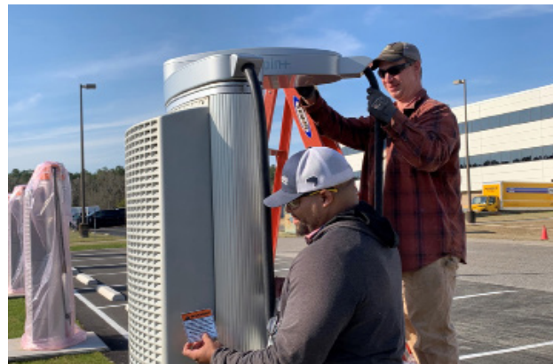
Savannah River Nuclear Solutions employee Alfonzo Thomas, left, helps Hebbard Electric electrician Greg Jamison prepare eight vehicle charging stations behind a building in the Savannah River Site’s B Area.
