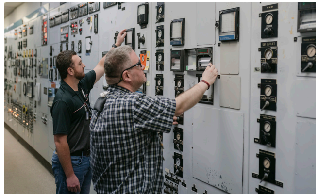
H Canyon Control Room operators Tyler Sullivan and Paul Gettle check First Uranium Cycle readings during its recent inactivation activities.
