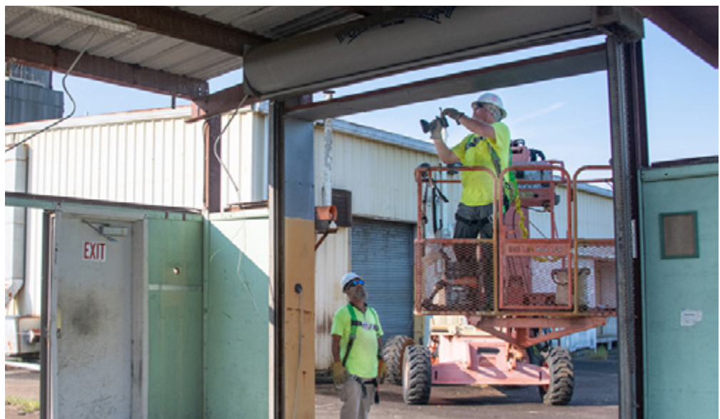
Subcontractor employees managed by Savannah River Nuclear Solutions work to dismantle one of six Savannah River Site buildings that will be donated to an organization created to support economic development initiatives throughout the region.
